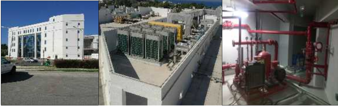
CCC New Head Quarter Building at Shati Al Qurum – MEP Installations
