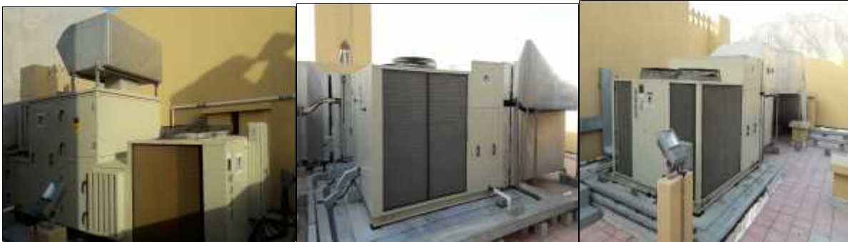
Sultan Qaboos Mosque at Bukha - HVAC Installations
