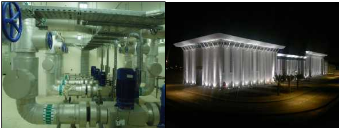
Royal Opera – Muscat - Store at Ghala - MEP Installations
